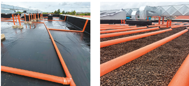
Collection piping made of PVC DN 110 before the placement of the filter layers (left), and distribution piping made of PP DN 110 together with perforated PP pipes (d40) on the filter surface, covered with halved PVC pipe profiles before being overlaid with a load-bearing layer of washed gravel (right).
