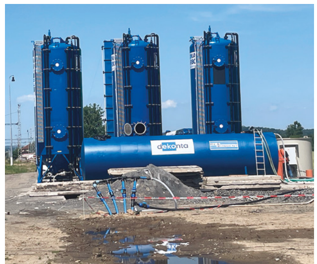
Large-capacity activated carbon filters
